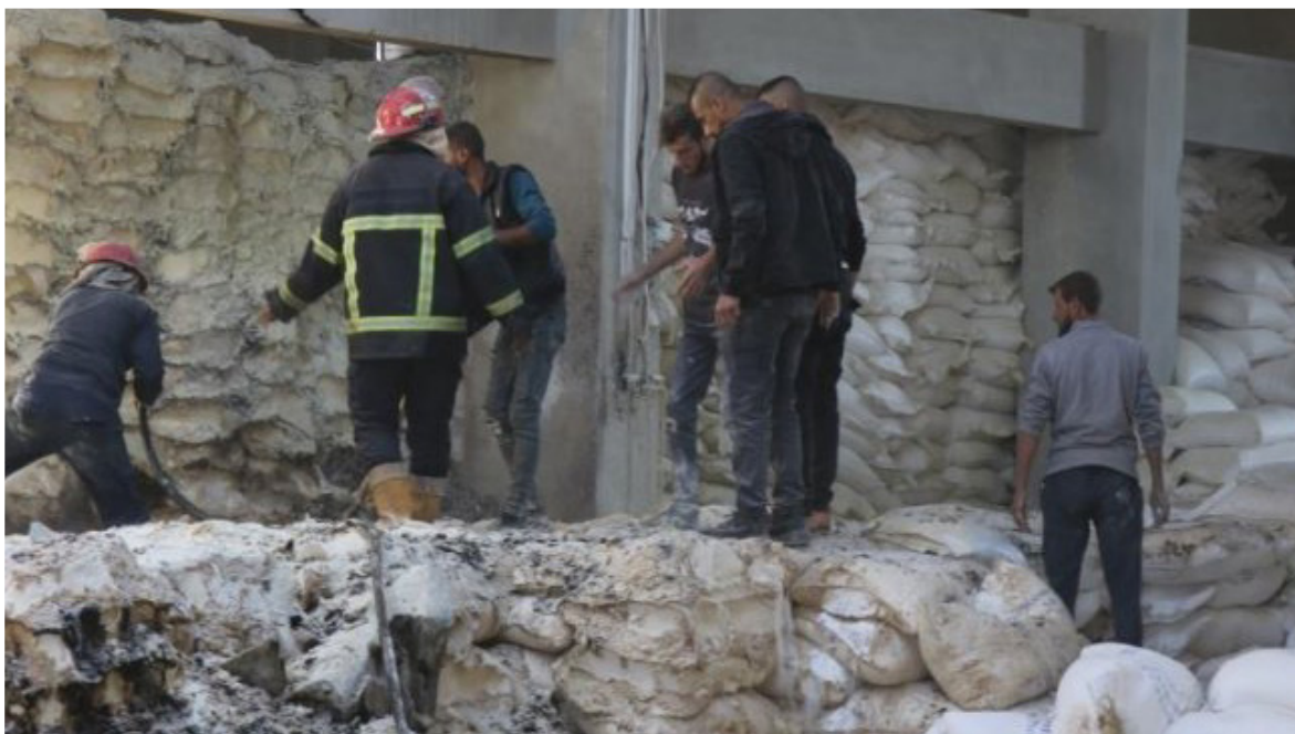
Grain silos bombed by Turkish drones in Qamishlo 24.10.2024 [Source: ANHA]
