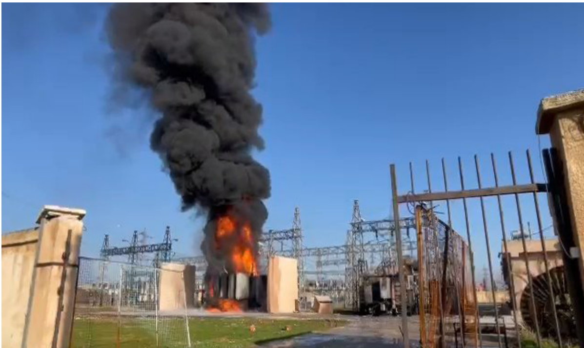
Qamishlo electricity station following Turkish airstrike, 15.01.2024
